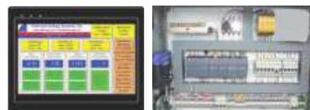
Typical Touch Screen Operator Interface. Siemens S7-1200 PLC with Ethernet Interface and DSL Router.
